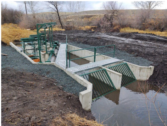
A three-bay rotary drum screen installed in the John Day River.
